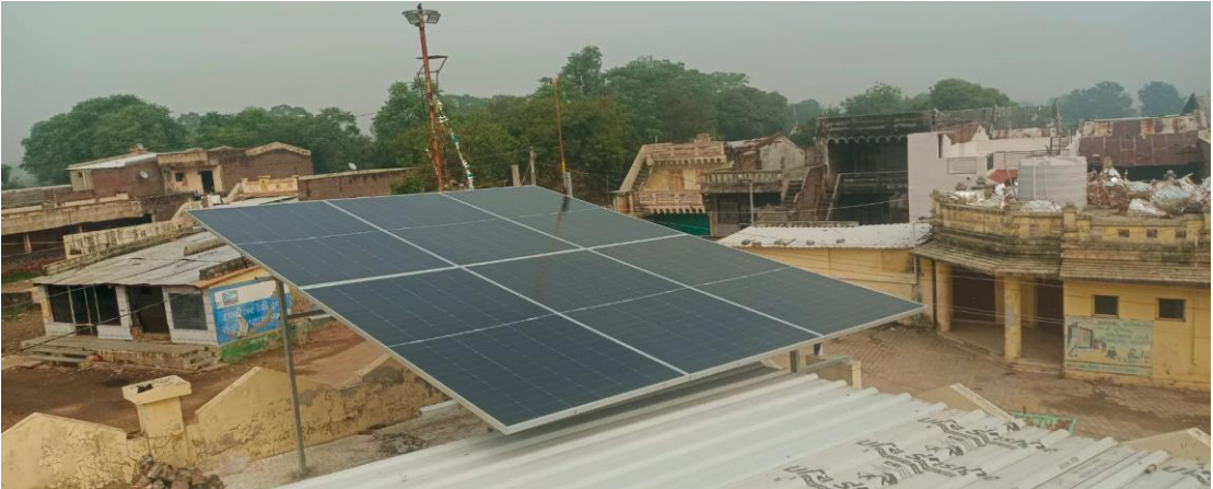
Installed solar panel at a village in Gujarat to promote green energy leading to savings in electricity cost
